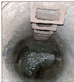
Three manholes had steel stairs so badly corroded that they fell off when hit with a hammer. Note water infiltration.
